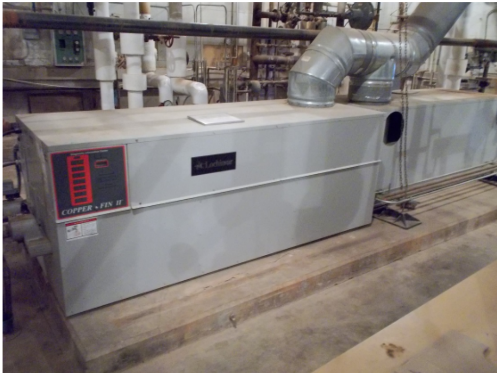
Existing Copper Fin Tube Gas Fired Boilers
