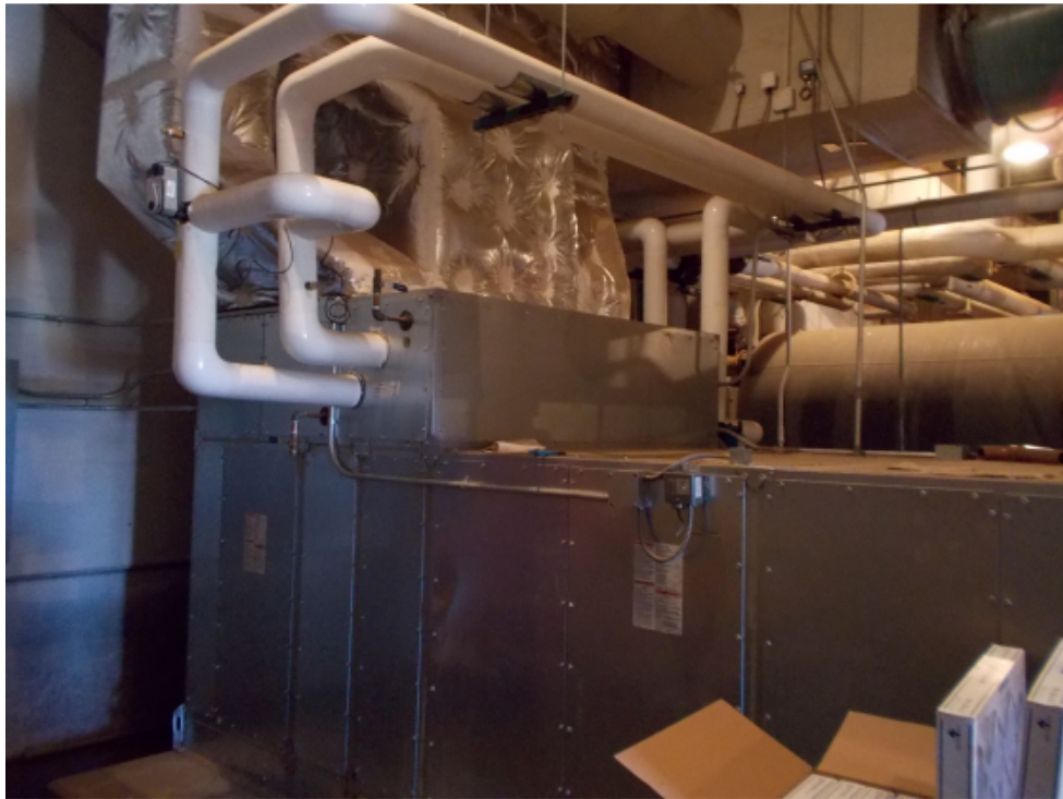
Typical Air Handling Units – Multizone Unit
