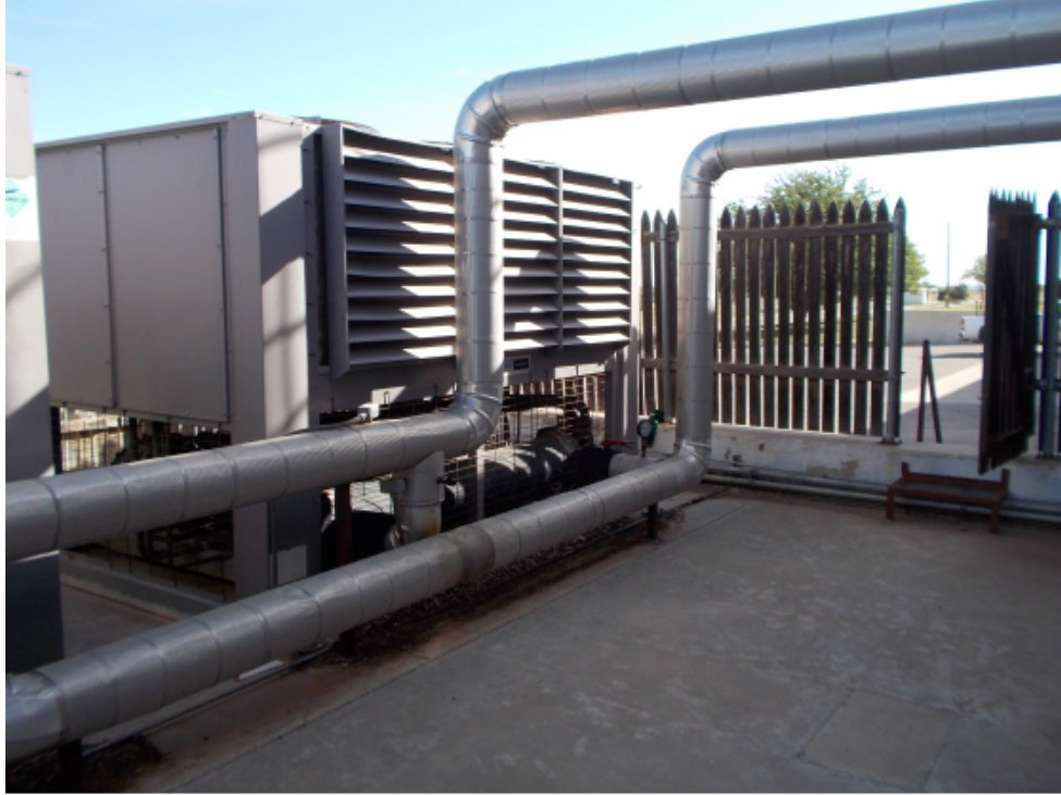
Existing Carrier Air Cooled Chiller
